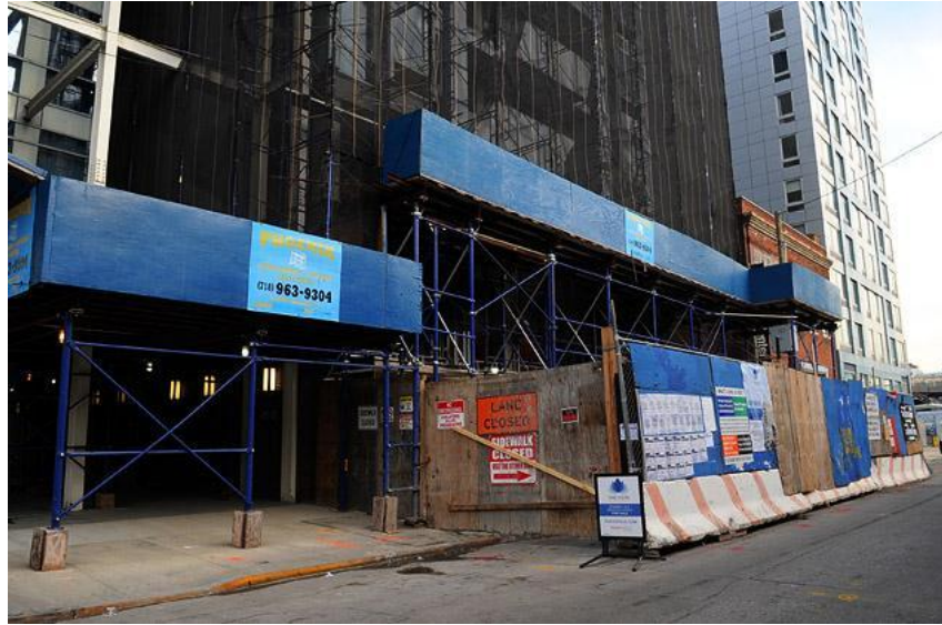
Construction on Purves St. in Long Island City is part of a residential boom.
