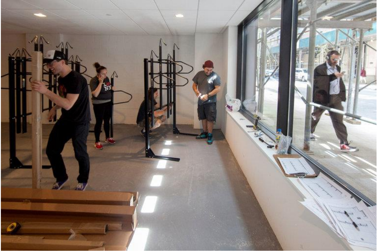
Bike storage racks are installed at 535W43, a luxury rental building nearing completion on West 43rd Street
