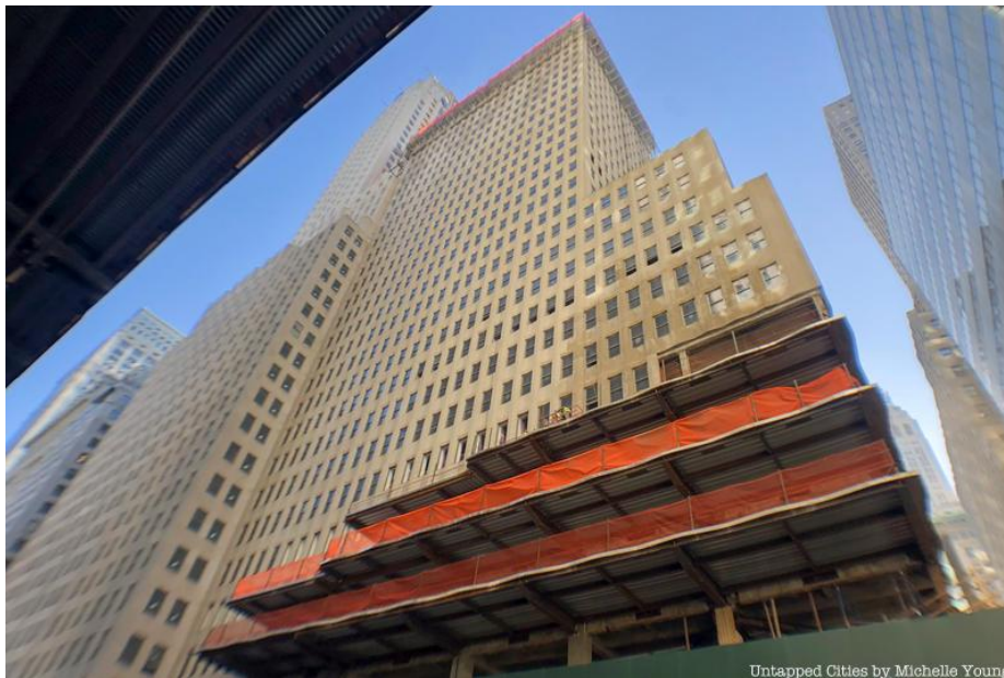
The 1963 extension of One Wall Street, with the new undulating glass facade under construction
