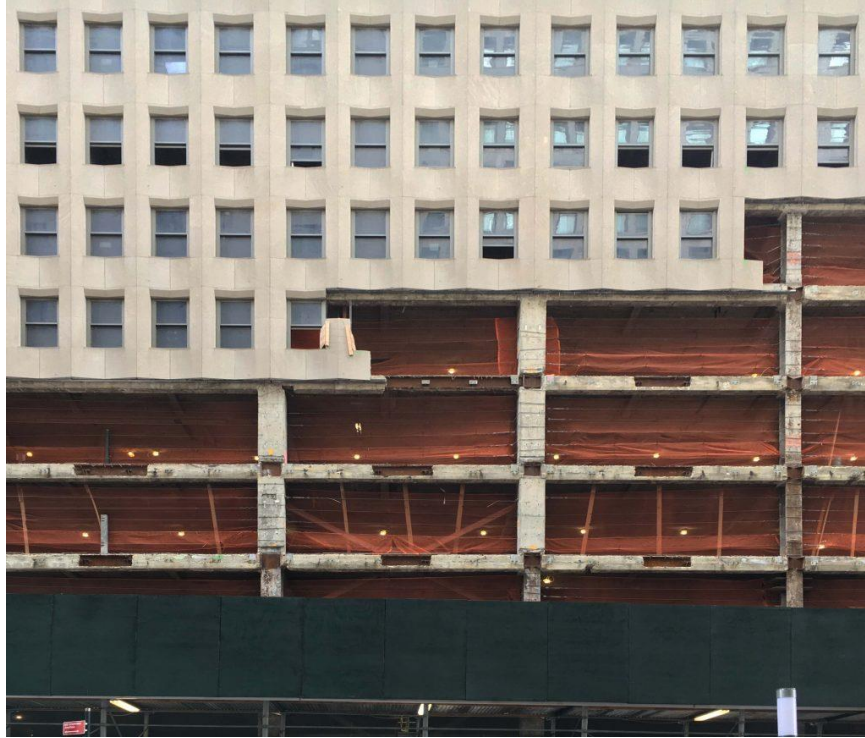
The facade of One Wall Street partially removed at and above street level to make way for the Whole Foods set to come. Photo by Michael Young
