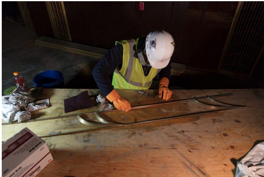
A worker cleaning and restoring one of the decorative ornaments that are part of the stylish and elegant window frames for the Red Room.
