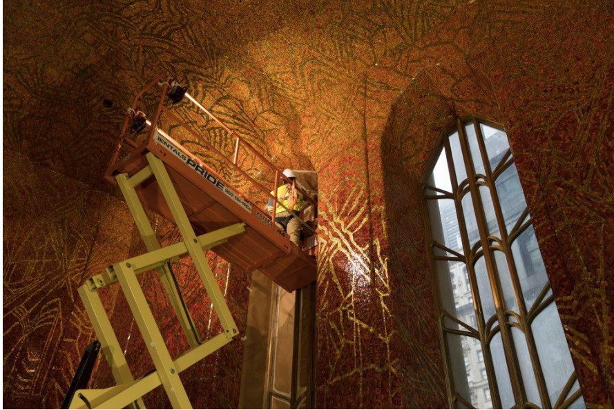
A worker using a scissor lift to reach the grand heights of the ceiling
