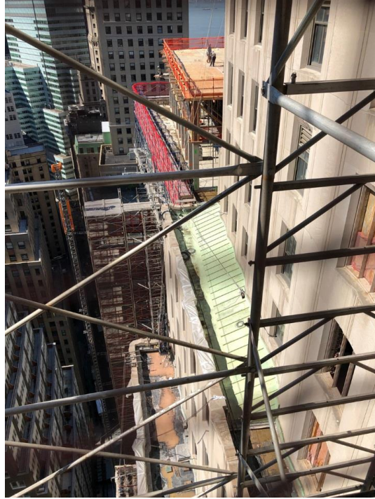
Looking through the mechanical hoist at the western elevation of One Wall Street. Photo by Michael Young
