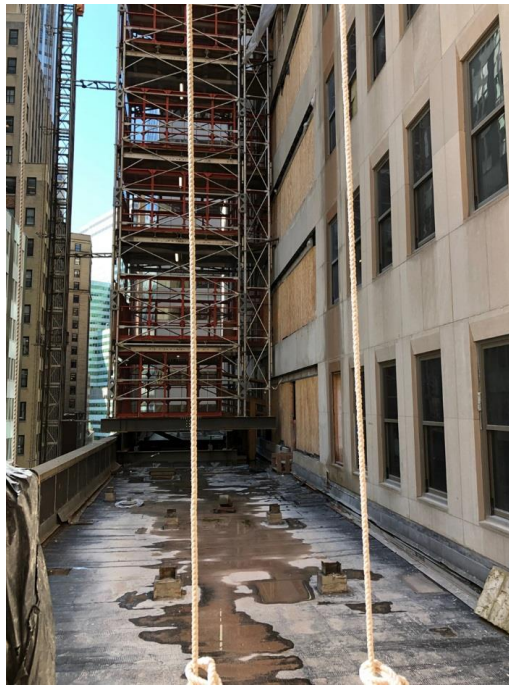
One of the lower setbacks and hoists on the western elevation. Photo by Michael Young
