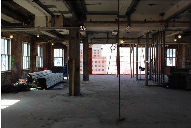
The floor-to-ceiling opening in the wall will eventually lead to the new addition of One Wall Street. Photo by Michael Young
