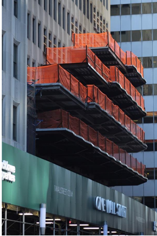
Looking south at the new protruding steel decking. Photo by Michael Young
