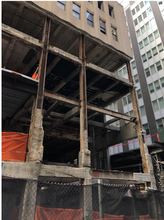
The corner of the southern elevation with the curtain wall removed, exposing the steel structure. Photo by Michael Young
