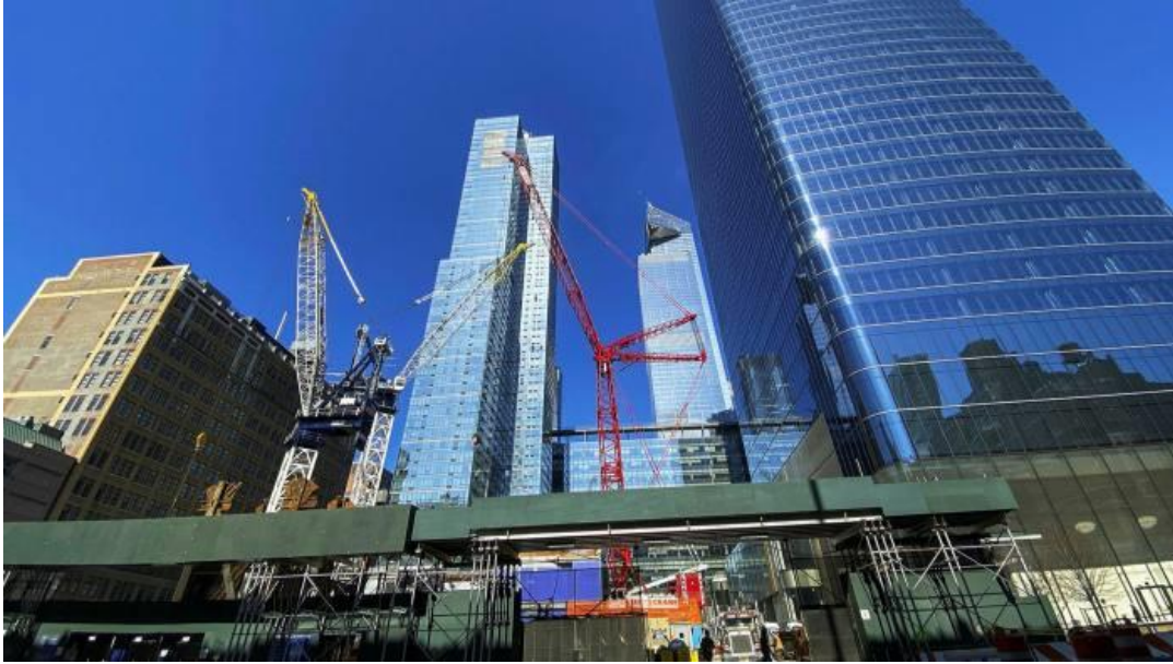
Several New York luxury developments are behind schedule because of the complexity of constructing a new generation of 'supertall' towers Eduardo Munoz Alvarez/ Getty
