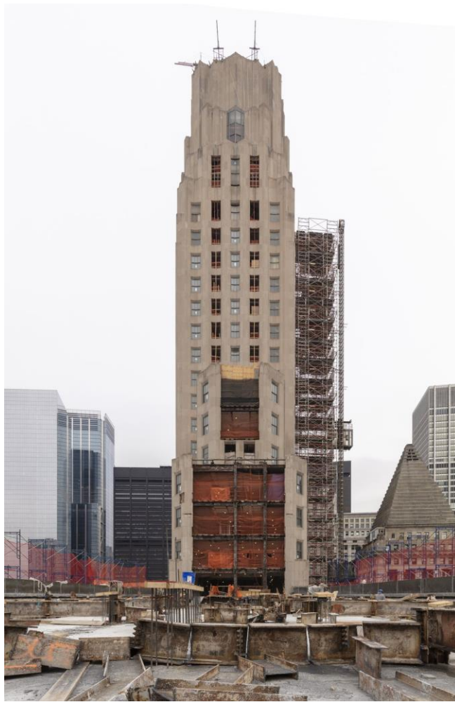
The tower portion, made from Indiana limestone, is largely untouched save for new windows. DBOX
