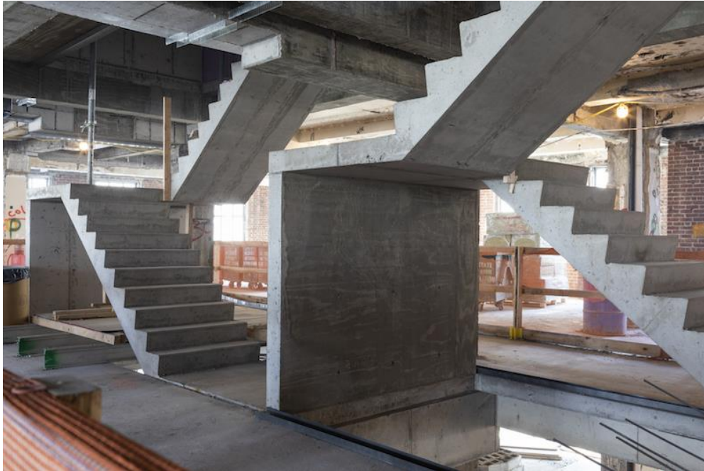
To free up more space, the Building Team moved the stairwell to the center of the building, and reduced the number of elevators to 10, form 34. Image: Courtesy of Macklowe Properties
